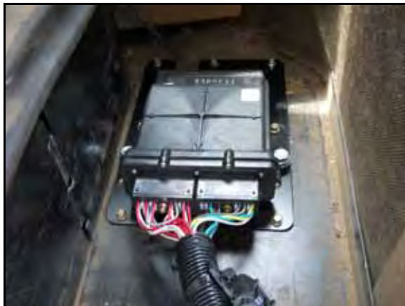
FIGURE 4. Node Harness Installed on Node
