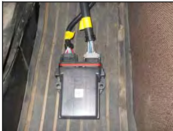
FIGURE 11. Node and Valve Harness Connected to Interface Box
