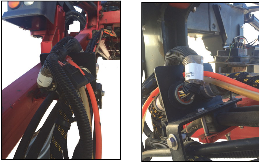
FIGURE 2. Miller N4 Interface Cable Connected to Machine Harness
