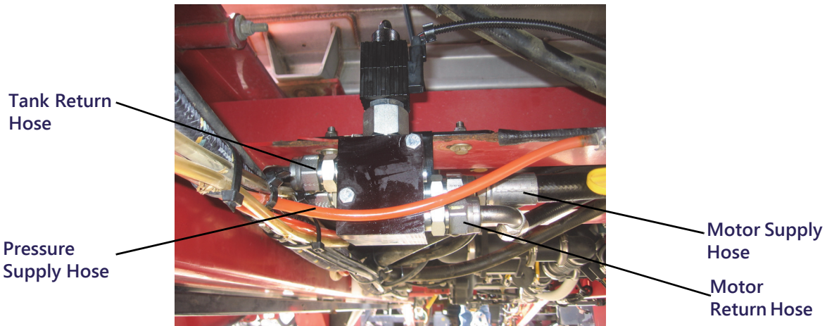
FIGURE 2. Installed PWM Valve
