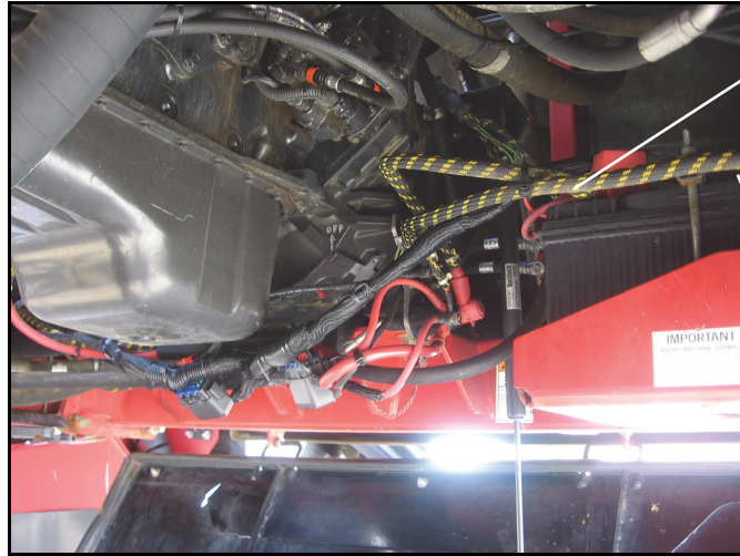
FIGURE 6. Installed Chassis and Nozzle Power Cables
