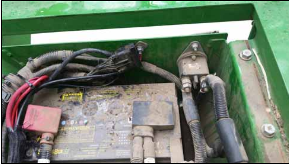
FIGURE 2. Grounded Chassis Cable and Hawkeye Power Cables
