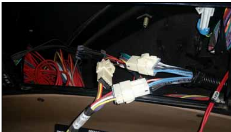
FIGURE 16. Tee Cable Connection
