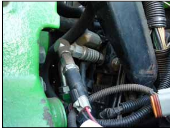
FIGURE 7. Transducer Assembly Installed on DR Port
