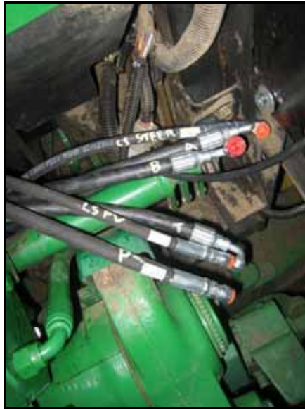
FIGURE 2. Routed Hoses to Valve Mounting Location
