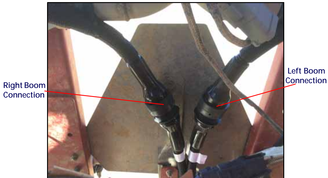
FIGURE 7. Boom Cable Connections
