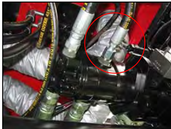
FIGURE 5. Machine's Existing Pressure Hose
