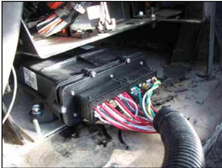
FIGURE 10. Node Cable Installed on Node
