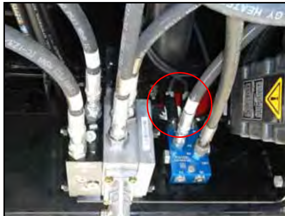
FIGURE 10. Valve Harness Connected to Flow Switch
