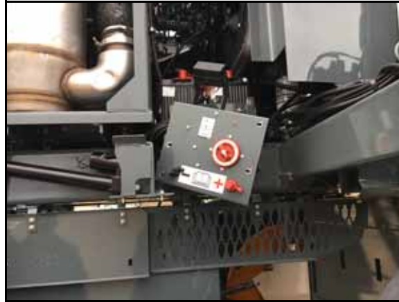
FIGURE 7. Battery Panel Cover Removed
