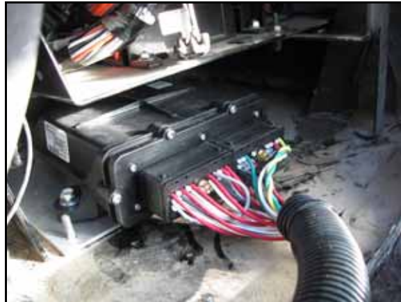
FIGURE 6. Node Harness Installed on Node
