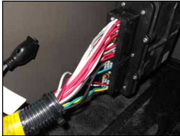
FIGURE 16. Node Harness Installed on Node
