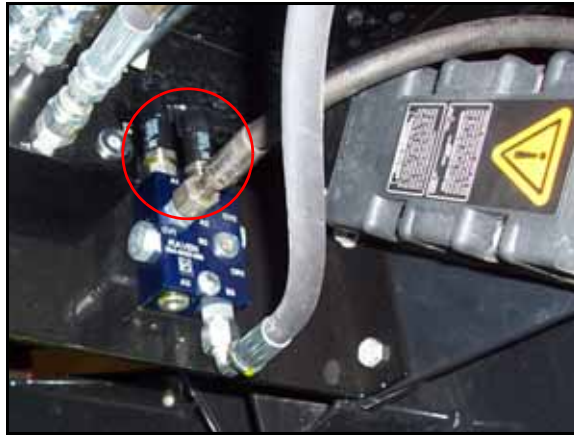
FIGURE 23. Valve Cable Connected to Flow Switch
