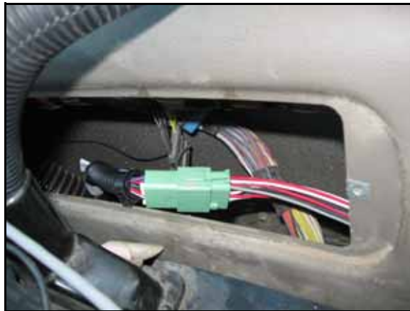
FIGURE 22. Valve Harness Connected to Node Harness
