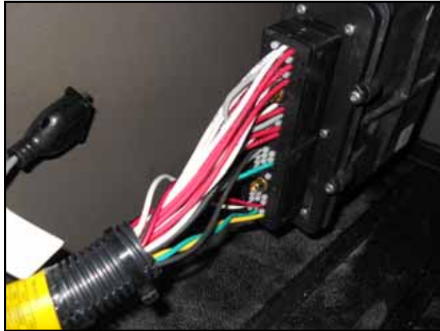
FIGURE 15. Node Harness Installed on Node
