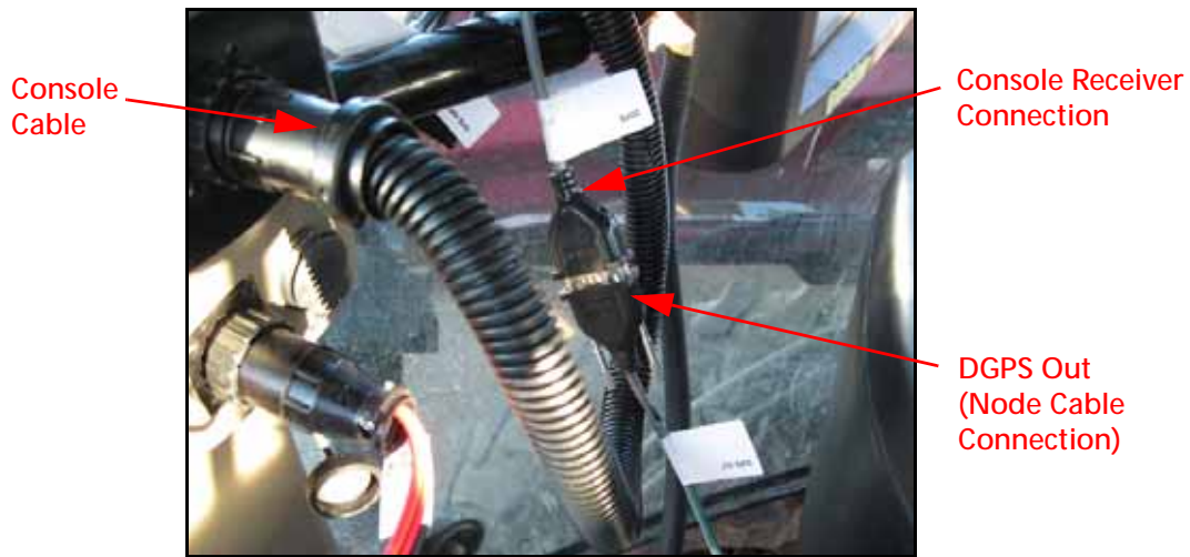
FIGURE 19. DGPS OUT Connected to Console Receiver Connection
