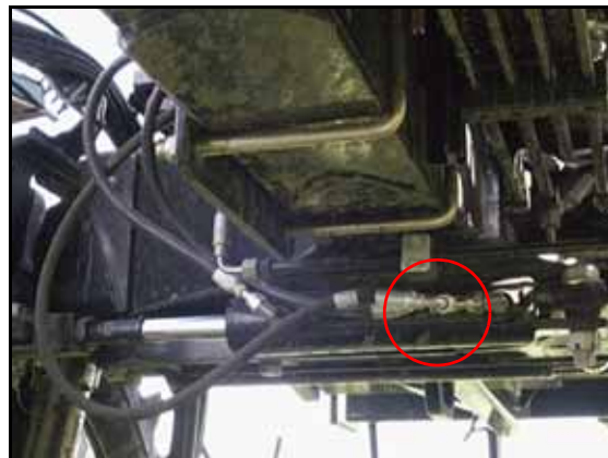
FIGURE 9. Right Steering Hose Installed
