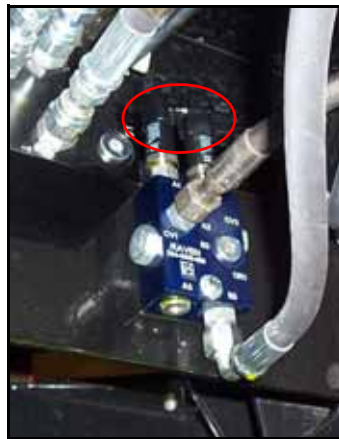
FIGURE 9. Valve Harness Connected to Flow Switch
