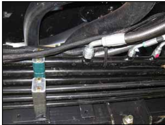
FIGURE 10. Machine's Steel Tank Line
