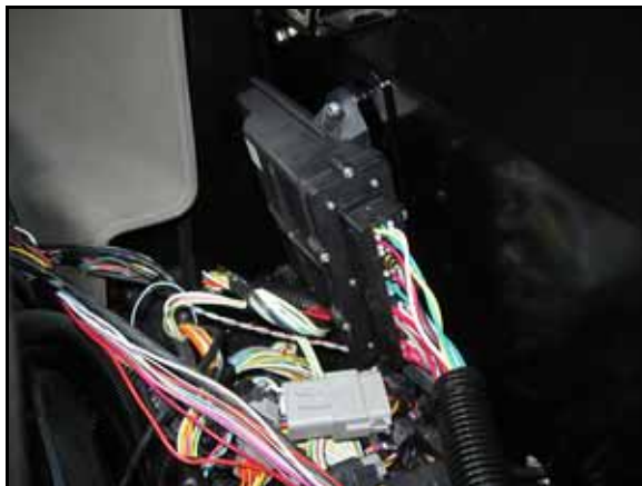
FIGURE 5. Node Harness Installed on the Node
