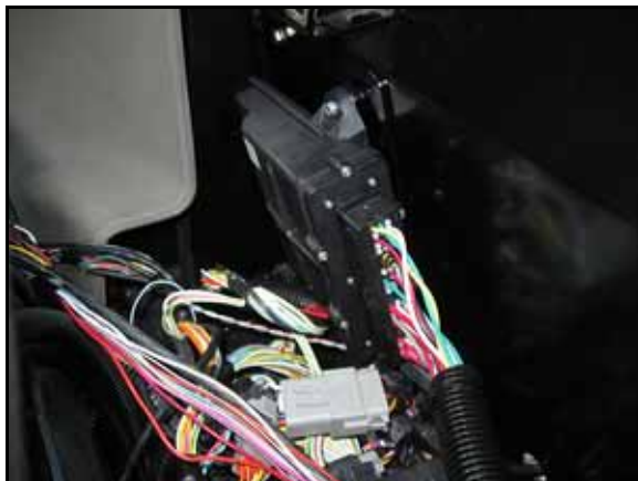
FIGURE 6. Node Harness Installed on the Node
