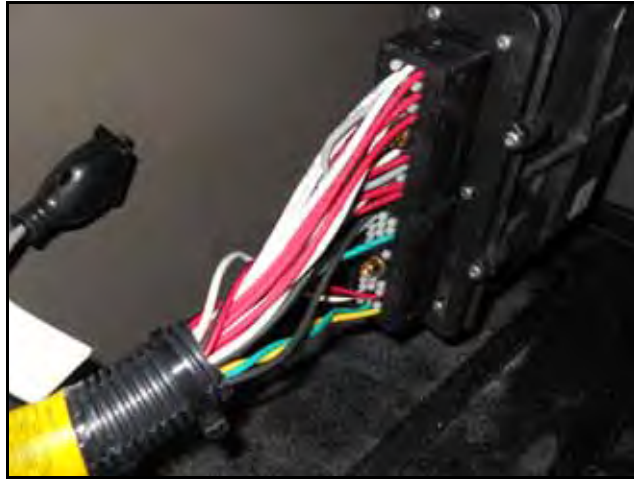
FIGURE 16. Node Harness Installed on Node
