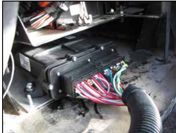
FIGURE 6. Node Harness Installed on Node
