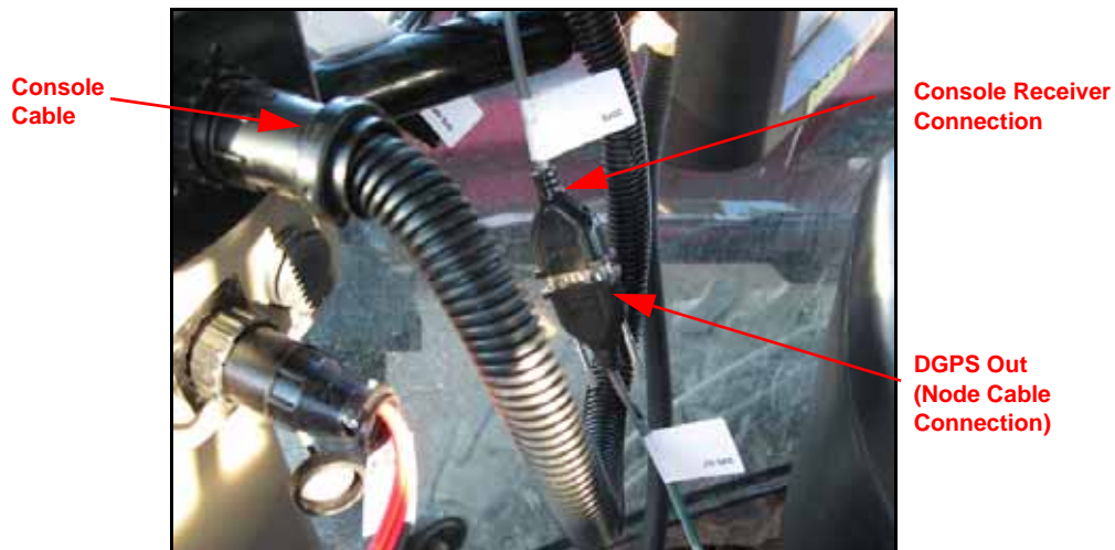
FIGURE 19. DGPS OUT Connected to Console Receiver Connection
