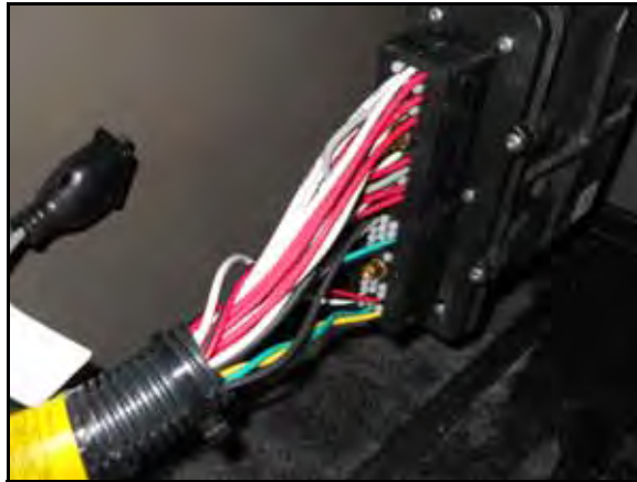
FIGURE 16. Node Harness Installed on Node
