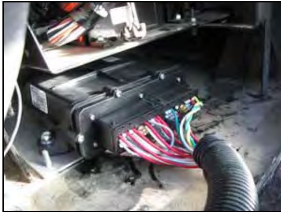
FIGURE 6. Node Harness Installed on Node
