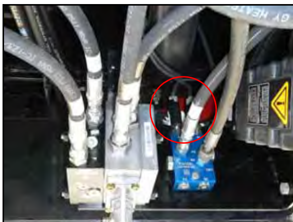
FIGURE 23. Valve Cable Connected to Flow Switch
