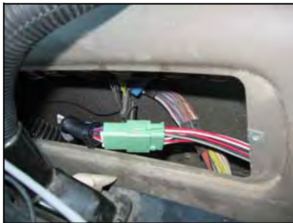
FIGURE 22. Valve Harness Connected to Node Harness
