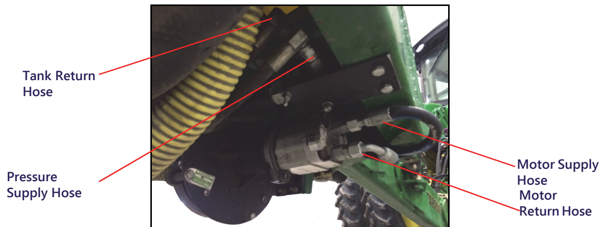
FIGURE 3. Installed PWM Valve
