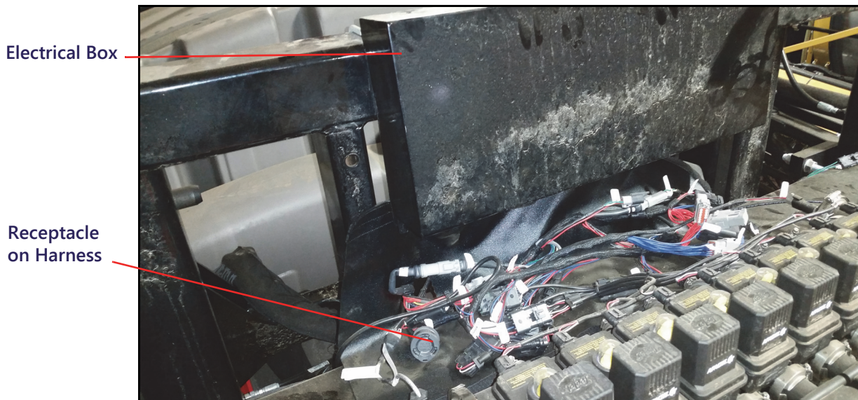
FIGURE 2. Harness Under Electrical Box
