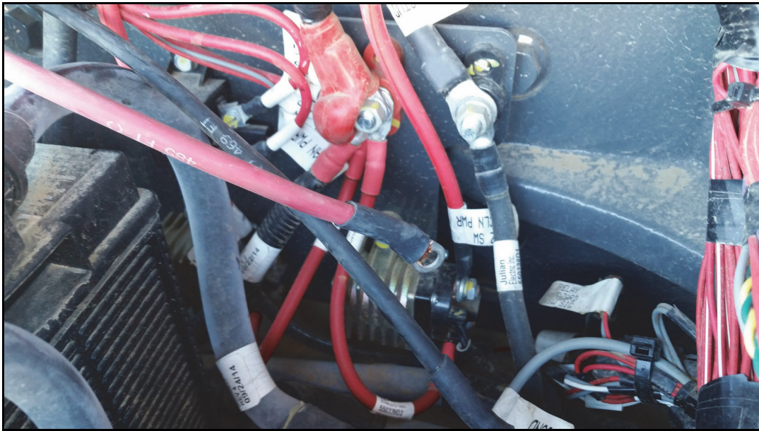
FIGURE 4. Battery Box Connections
