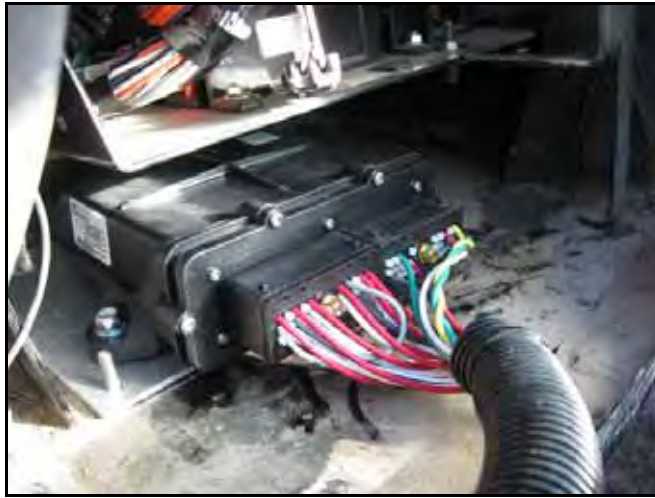
FIGURE 6. Node Harness Installed on Node
