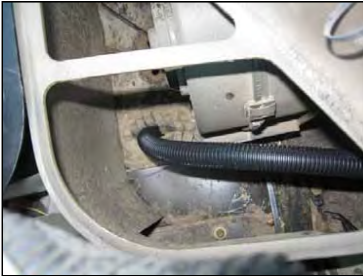
FIGURE 13. Valve Cable Routed Through Access Point
