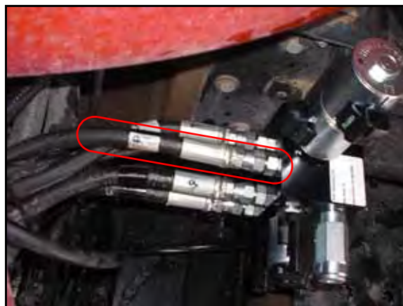
FIGURE 9. Pressure Hose Installed on SmarTrax Valve
