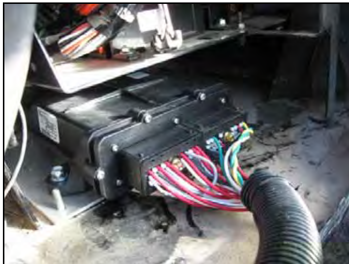
FIGURE 8. Node Cable Installed on Node
