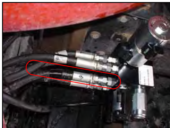
FIGURE 5. Left Steering Hose Installed on SmarTrax Valve
