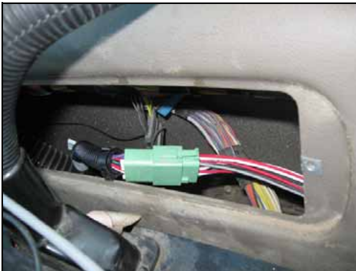
FIGURE 14. Valve Harness Connected to Node Harness
