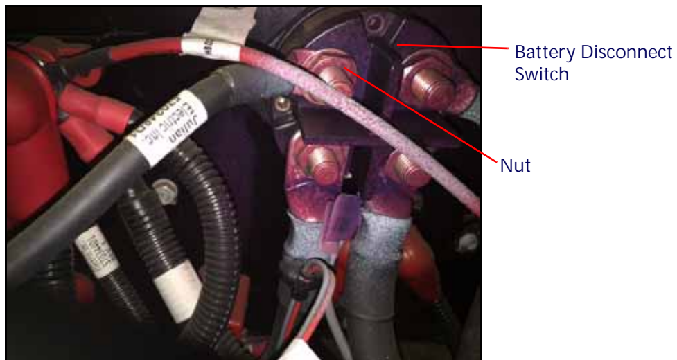
FIGURE 6. Battery Disconnect Switch
