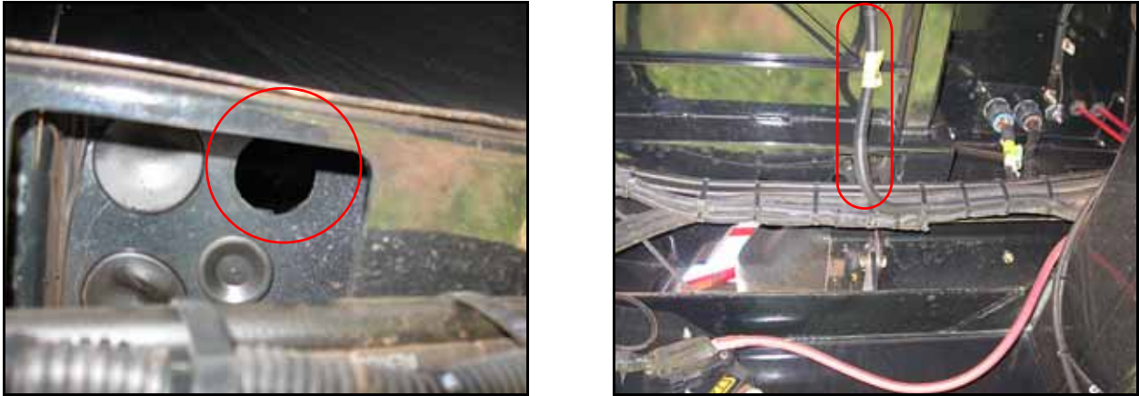
FIGURE 10. Valve Harness Routed Outside of the Cab
