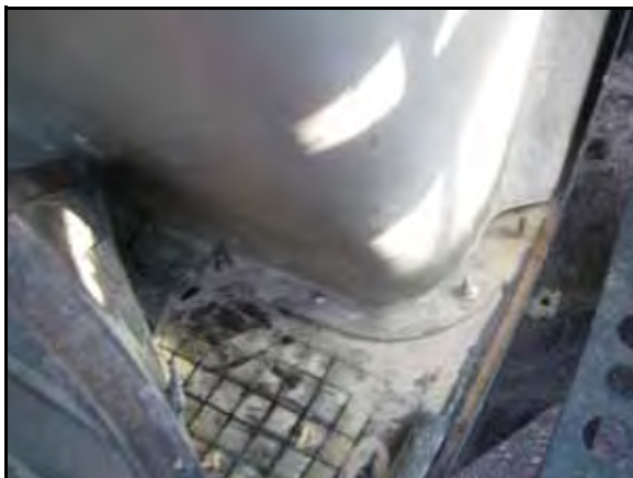
FIGURE 2. Floor Mat Removed from Cab
