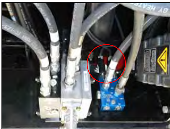
FIGURE 14. Valve Cable Connected to Flow Switch
