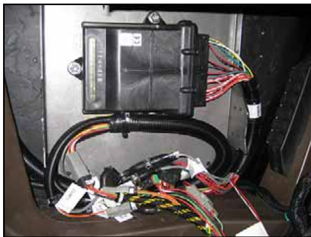
FIGURE 6. Final SmarTrax Node Installation
