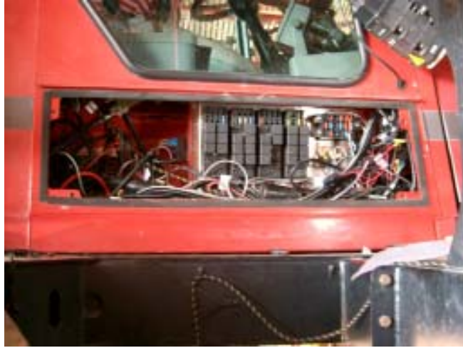
Switched Power Access Panel
