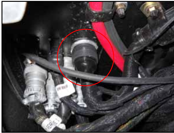
FIGURE 9. Valve Harness Secured to Bulkhead
