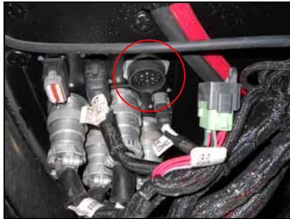
FIGURE 7. Node Harness Secured to Bulkhead
