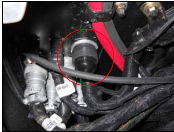
FIGURE 9. Valve Harness Secured to Bulkhead
