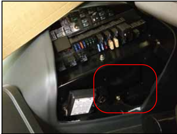
FIGURE 1. SmarTrax Node Mounting Location - Side Console Panel Removed
