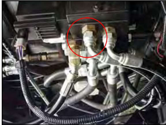
FIGURE 13. Hydraulic Hose Installed on SmarTrax Valve
