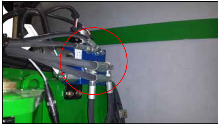
FIGURE 1. Hydraulic Valve Installed
