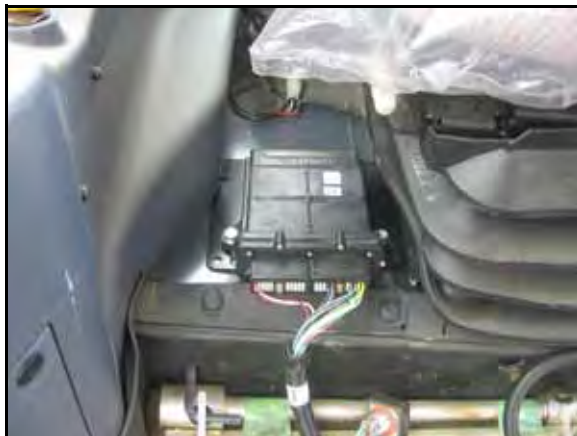
FIGURE 5. Node Harness Installed on the SmarTrax MD Node
