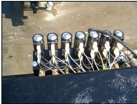
FIGURE 2. Machine's Boom Function Coils
