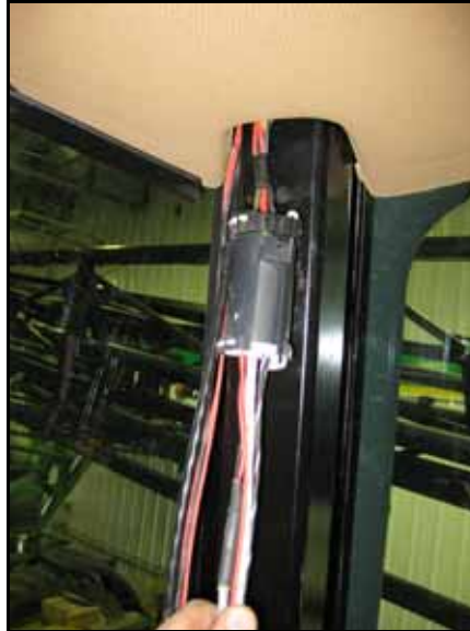
FIGURE 11. AutoBoom Harness Cable Connected
