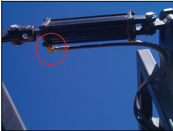
FIGURE 12. Cylinder Hoses Installed
