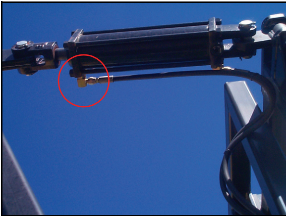
FIGURE 6. Cylinder Hoses Installed
