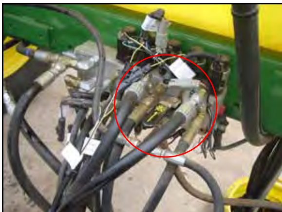
FIGURE 12. Left and Right Cylinder Hoses Installed
