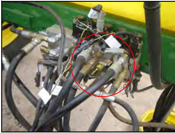
FIGURE 6. Left and Right Cylinder Hoses Installed
