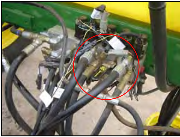
FIGURE 6. Left and Right Cylinder Hoses Installed
