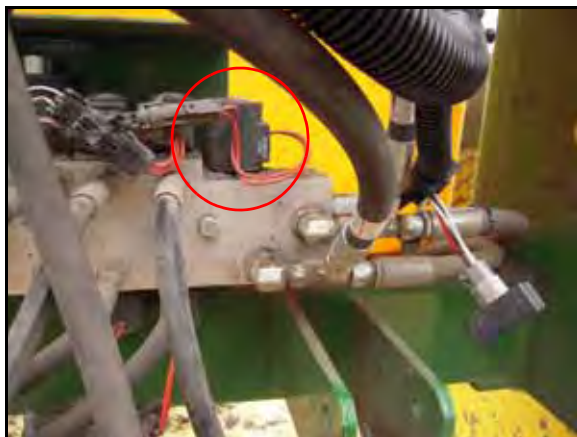
FIGURE 11. Directional Valve Boom Sense Adapter Cables Installed
