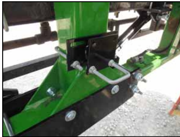
FIGURE 19. Cylinder Hose Retaining Bracket Assembly Installed
