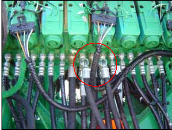
FIGURE 8. Down Hoses Installed on the AutoBoom Valve
