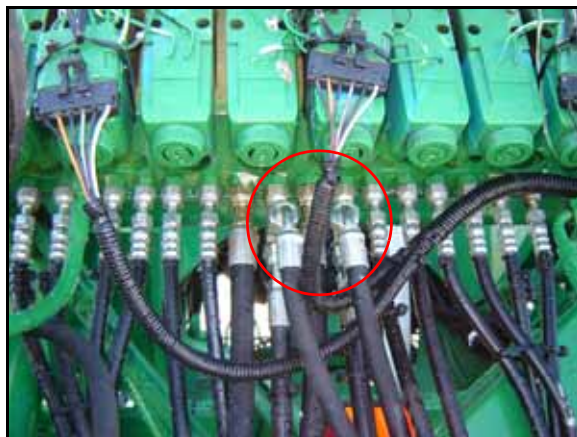
FIGURE 20. Down Hoses Installed on the AutoBoom Valve
