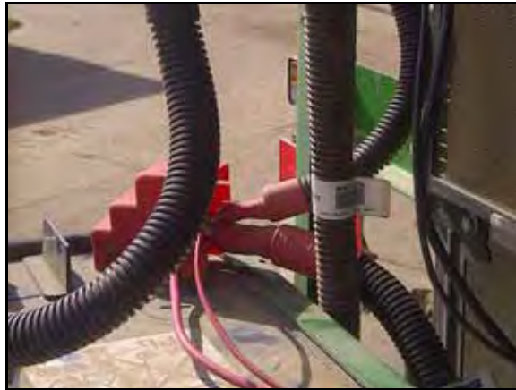
FIGURE 6. Power and Ground Wires Installed on Battery
