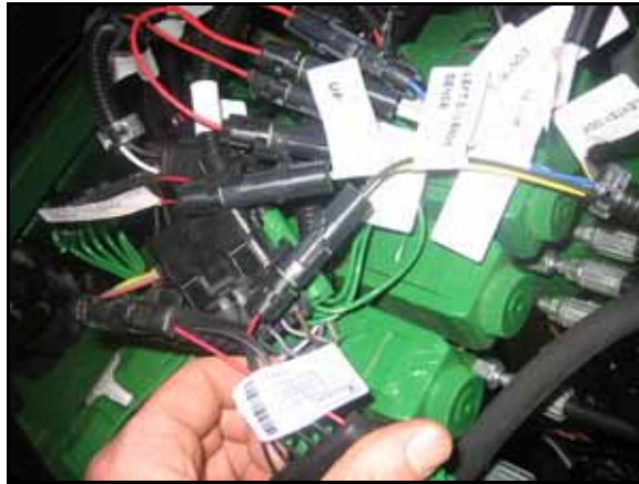
FIGURE 11. Machine's Boom Function Coils
