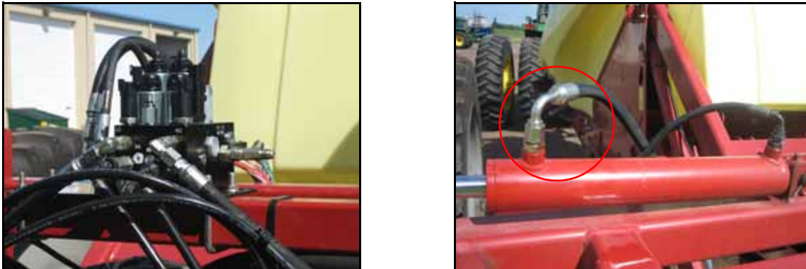
FIGURE 11. Cylinder Hoses Installed
