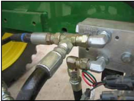
FIGURE 4. Pressure and Tank Hoses Installed
