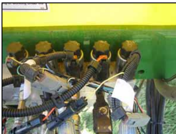
FIGURE 11. Boom Sense Adapter Cables Installed
