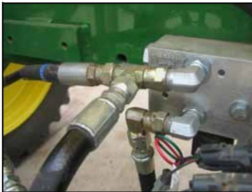
FIGURE 4. Pressure and Tank Hoses Installed
