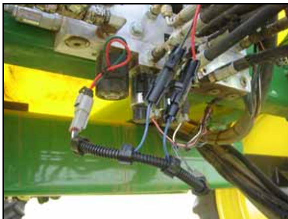
FIGURE 15. Center Rack Control Boom Sense Adapter Cable Installed
