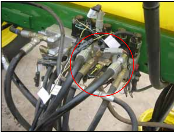
FIGURE 5. Cylinder Hoses Installed
