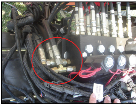
FIGURE 3. Pressure and Tank Hoses Installed
