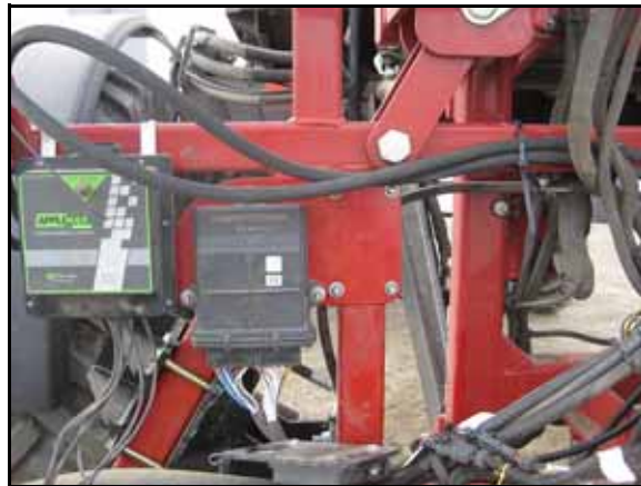
FIGURE 2. Hydraulic Sense Node Removed from Mounting Bracket
