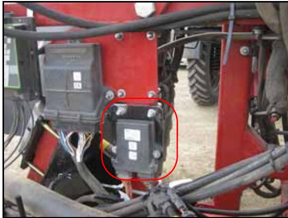
FIGURE 3. Hydraulic Sense Node Installed on Mounting Bracket
