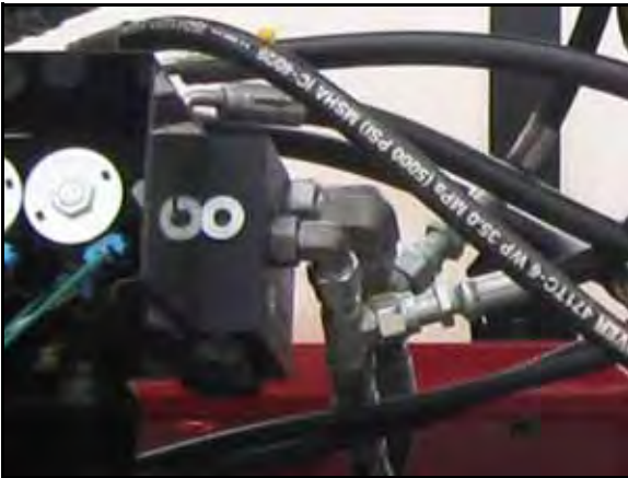
FIGURE 9. Pressure and Tank Hoses Installed
