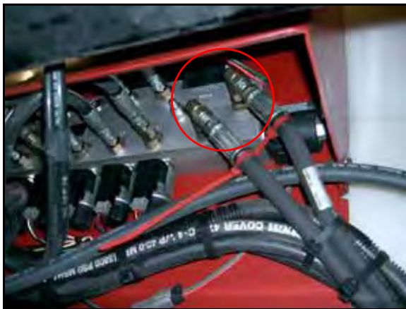
FIGURE 4. Pressure and Tank Hoses Installed
