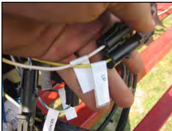
FIGURE 15. Machine's Up Cylinder Wiring
