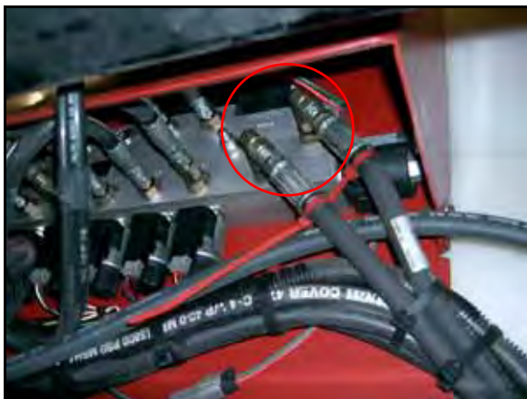
FIGURE 10. Pressure and Tank Hoses Installed
