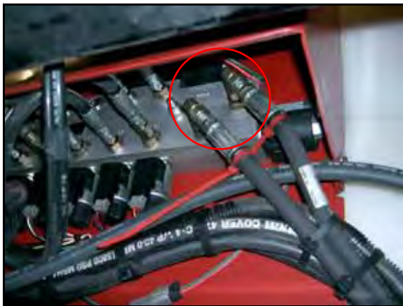
FIGURE 4. Pressure and Tank Hoses Installed
