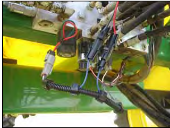
FIGURE 16. Center Rack Control Boom Sense Adapter Cable Installed
