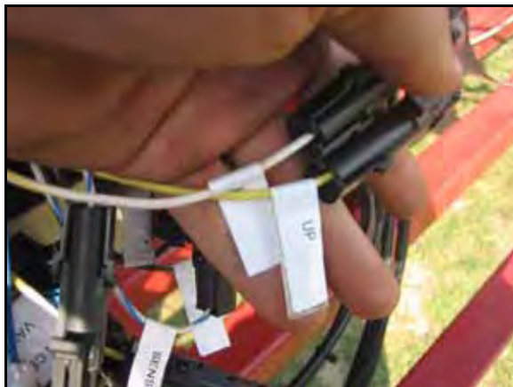
FIGURE 13. Machine's Up Cylinder Wiring
