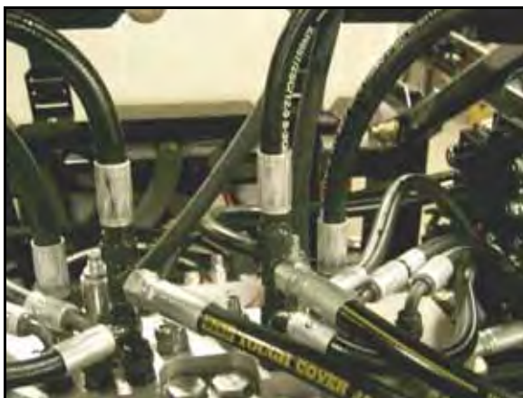
FIGURE 10. Left and Right Cylinder Hoses Installed
