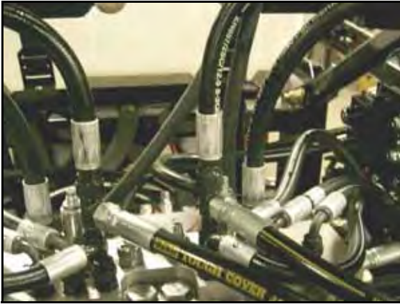
FIGURE 4. Left and Right Cylinder Hoses Installed
