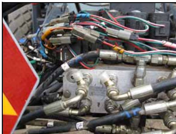
FIGURE 8. Machine's Down Hoses Installed on Tee Fittings
