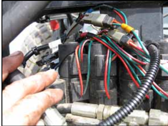
FIGURE 14. Machine's Left and Right Tilt Boom Function Coils
