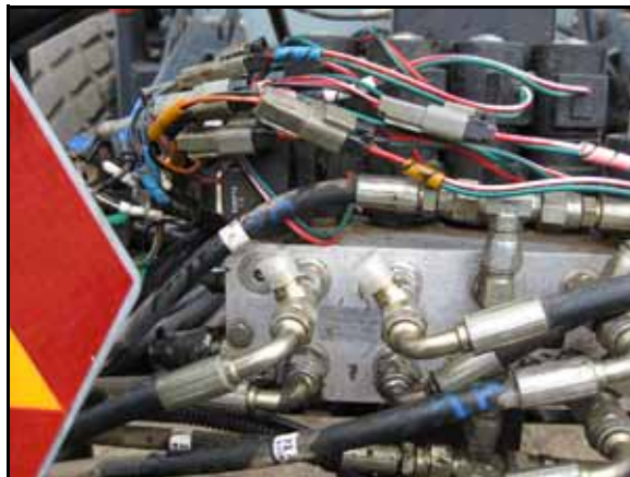
FIGURE 14. Machine's Down Hoses Installed on Tee Fittings
