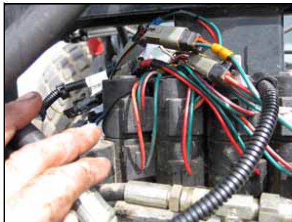
FIGURE 10. Machine's Left and Right Tilt Boom Function Coils
