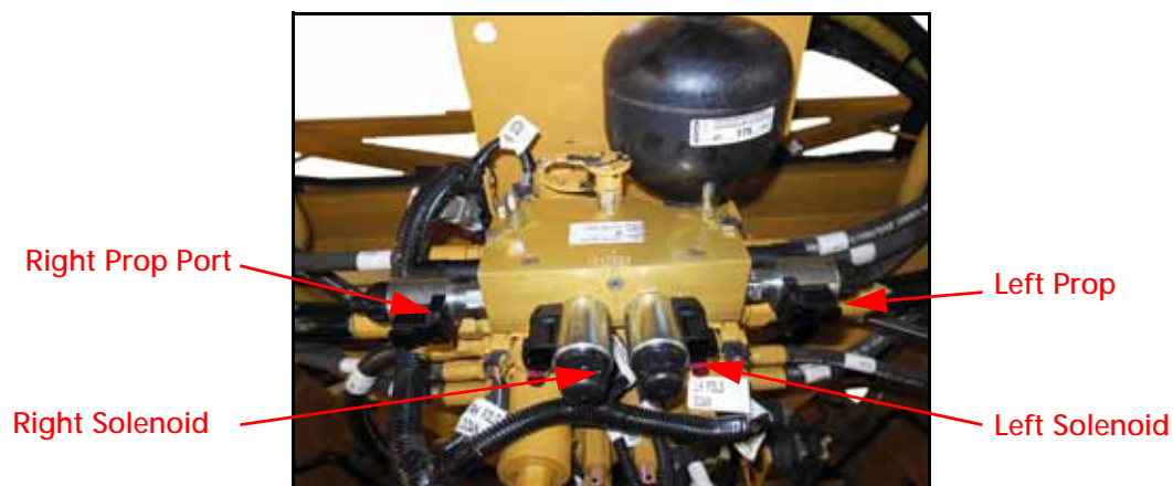
FIGURE 23. Harness Cabling Connections
