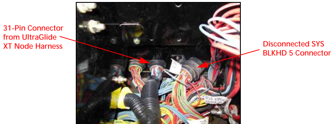
FIGURE 8. Node Harness Installed on Bulkhead (View from Inside Box)
