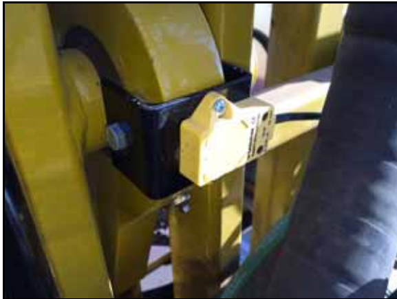
FIGURE 10. Rotary Sensor Installed
